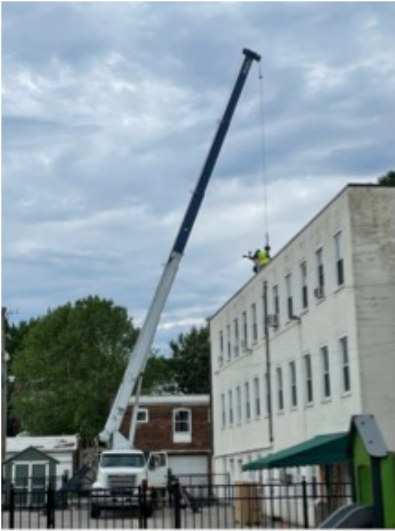
Vincent is in the yellow vest, helping secure the new equipment on the Williams Building roof.
